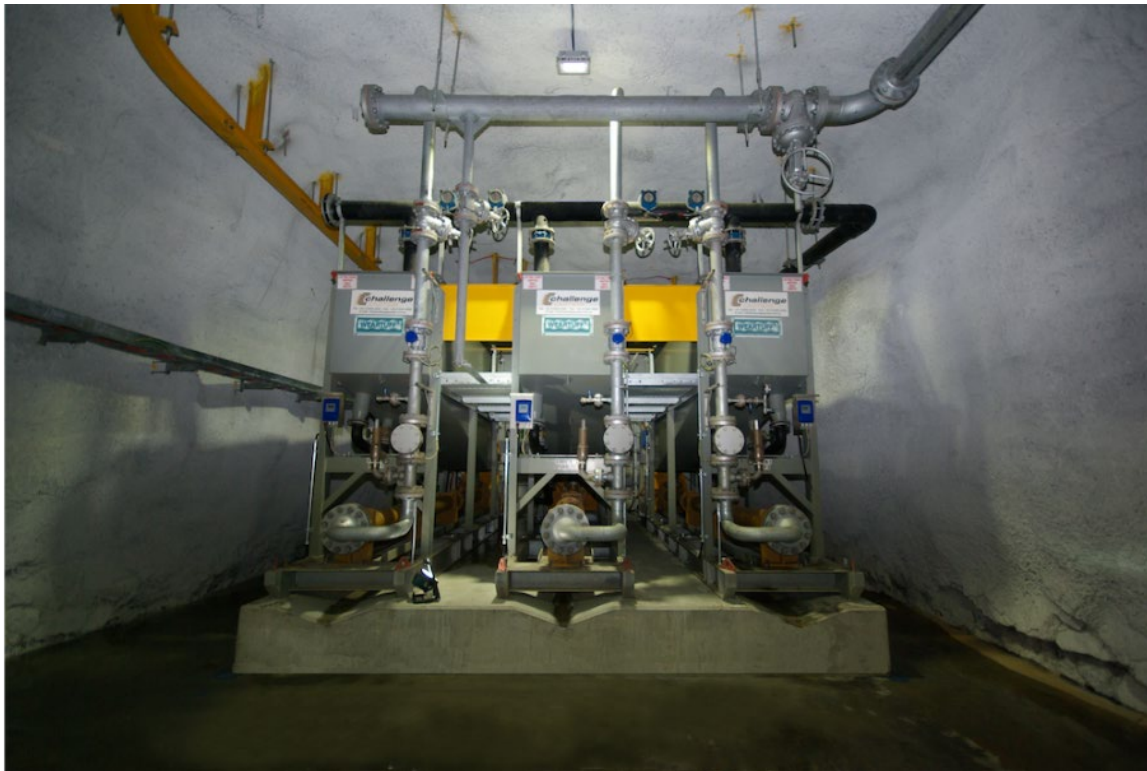
Figure 16.76: Photo of a Typical Underground Pump Station with Capacity of 60 L/s (Challenge Pumps Pty Ltd)
