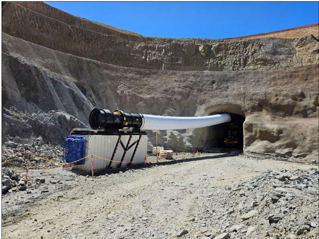
Figure 16.56: Photo of an Auxiliary Fan mounted on a Support Structure (Mintek Australia Pty Ltd)
